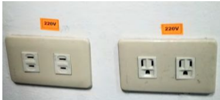
Fig. 3: Wall sockets in the Philippines are 220V
