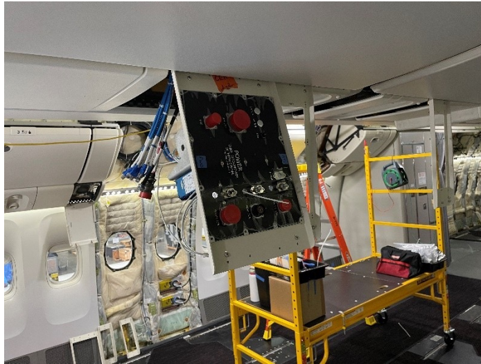
The new experimenter interface panel installed on the NASA B777. Credit: Derek Rutovic / NASA
